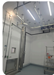
Hanging cooler storage
