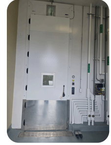
Utility runs & sanitary vent
